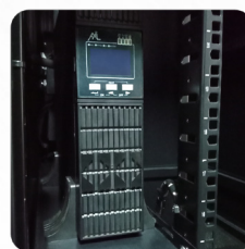
UPS Back-up Power
