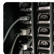
PDU Power Distribution Unit
